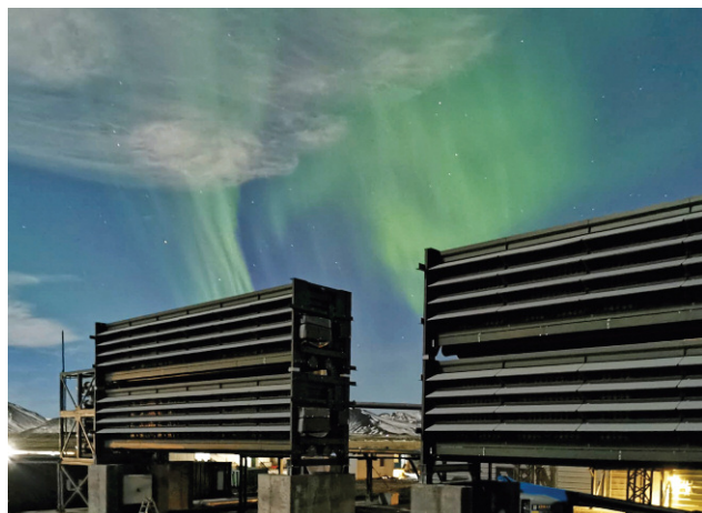
The Orca plant in Iceland, equipped with machines designed to reduce atmospheric levels of CO 2 by absorbing this greenhouse gas and storing it back underground.
